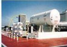
LCNG station within LA Airport
